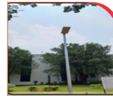
Solar street light @ U2
