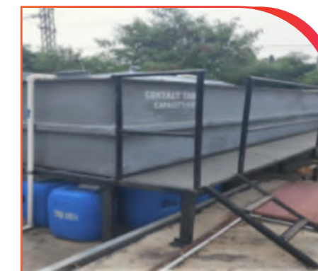
Effluent pre-treatment facility @NRM
